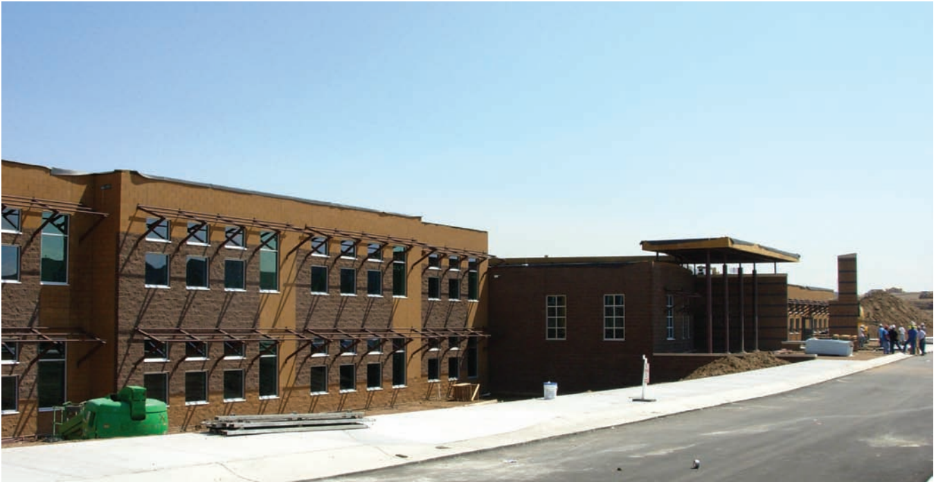
Stone Mountain Elementary near Denver is part of a school district that uses Web-based BACnet systems for most of its buildings.
