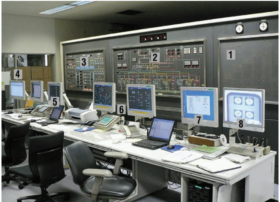
Photo 1: Operator workstations and remote stations of the building automation and control system: 1) mimic graphical panel for elevator system; 2) mimic graphical panel for power supply system; 3) mimic graphical panel for HVAC system; 4) BACnet operator workstations (B-OWS) for central plant operating support; 5) B-OWS for HVAC system; 6) B-OWS for power supply system; 7) B-OWS for building management system; and 8) closed-circuit TV.
